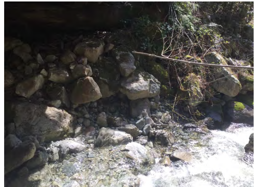
Downstream left bank erosion
