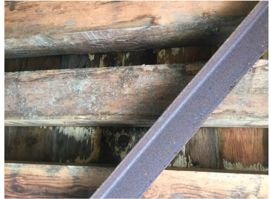
Indications of subdeck rot - cored and still in fair condition
